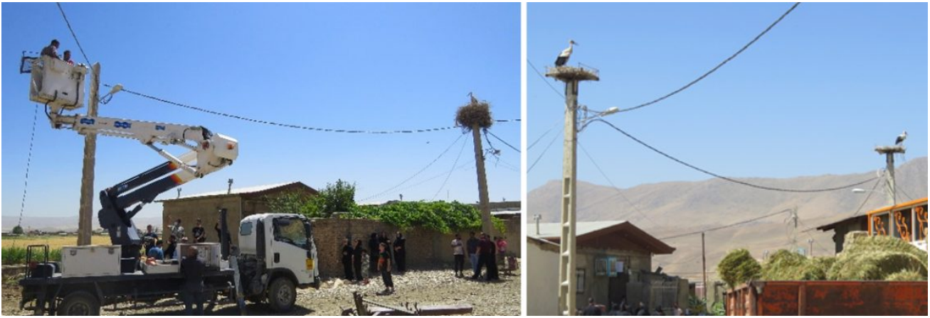
Left: nest platform installation. Right: white storks perching on the nest platforms. Photos: Mahmood Kolnegari.
